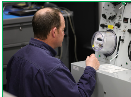
Nathan Klindt, metering superintendent, energizes a meter to get readings and check the display.
