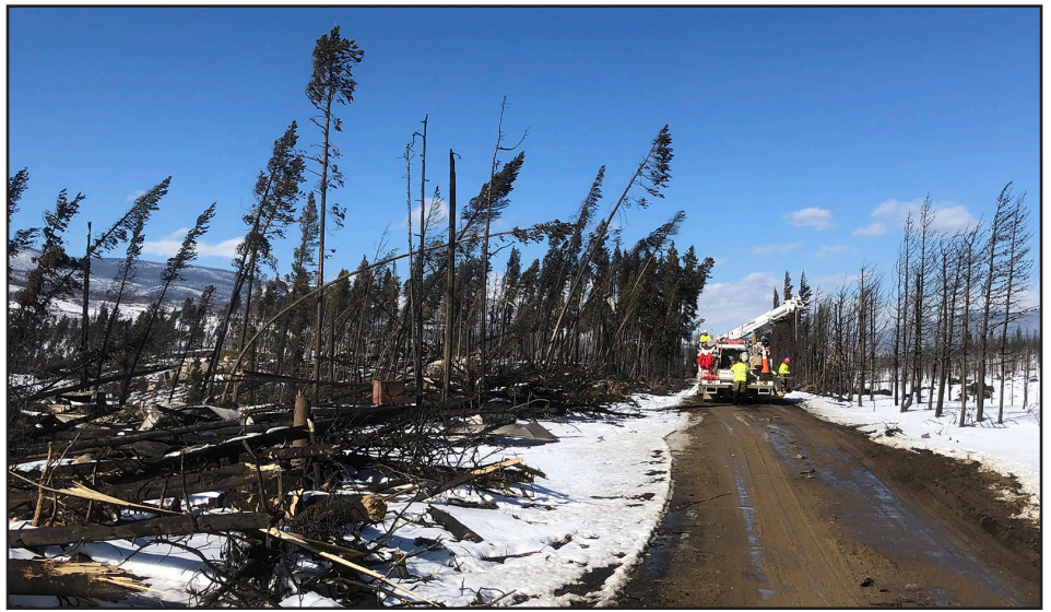
A mutual aid United Power crew joined MPE crews in rebuilding lines near Sun Valley, one of the hardest hit areas where the fire storm generated wind speeds over 110 miles per hour.
